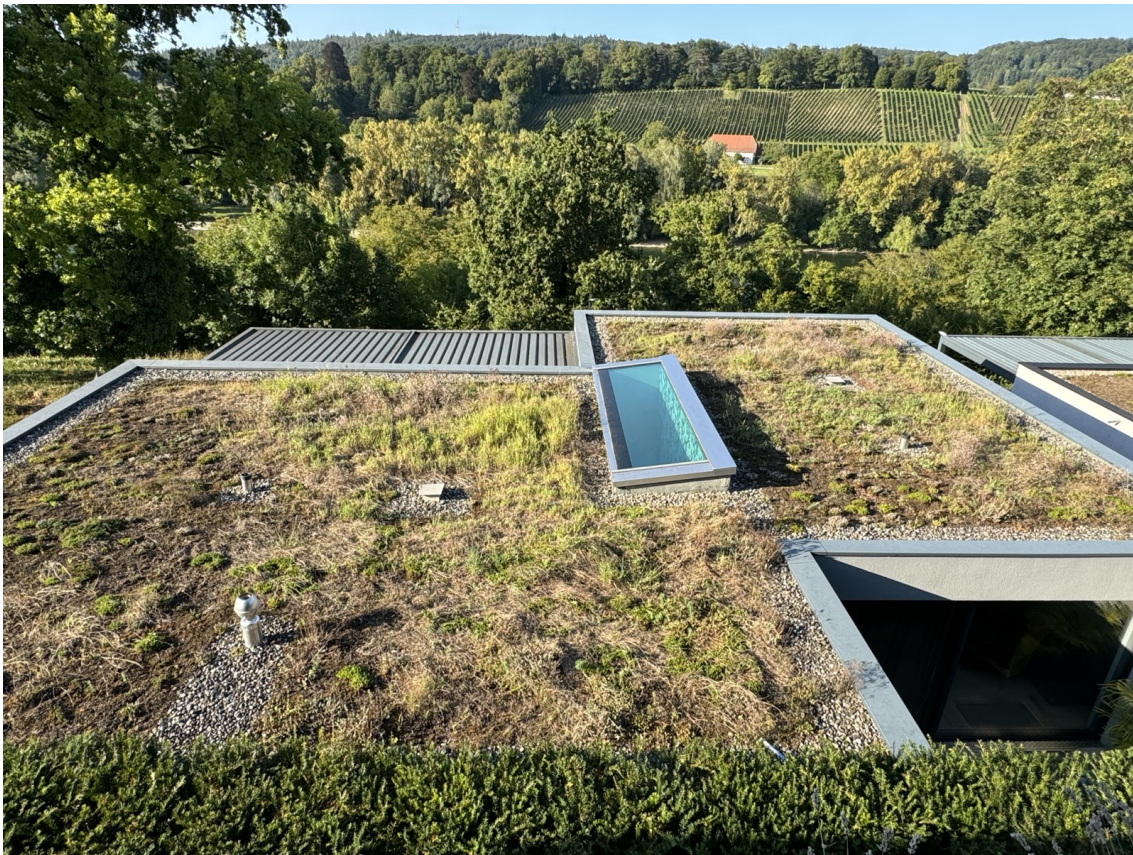
Figure 6.2: A green roof reduces the runoff and provides space for plants and insects. (Image: Martin Weber)
