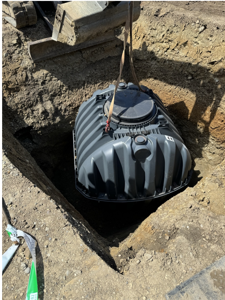
Figure 6.3: A rain water barrel placed into the garden. It stores 6500 L of water which is enough to water the garden for two weeks during a drought. (Image: Martin Weber)
