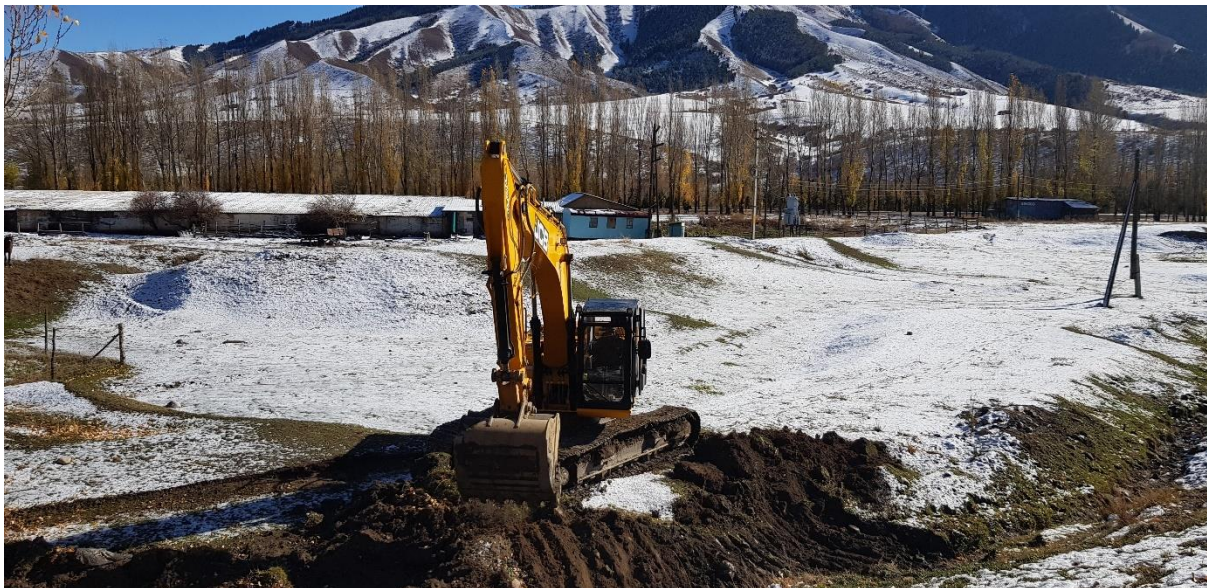
Figure 4: newly acquired excavator of the RWMD, where a canal that was difficult to maintain was finally fixed in Teploklyuchenka. Picture taken by author, 20.10.2023
