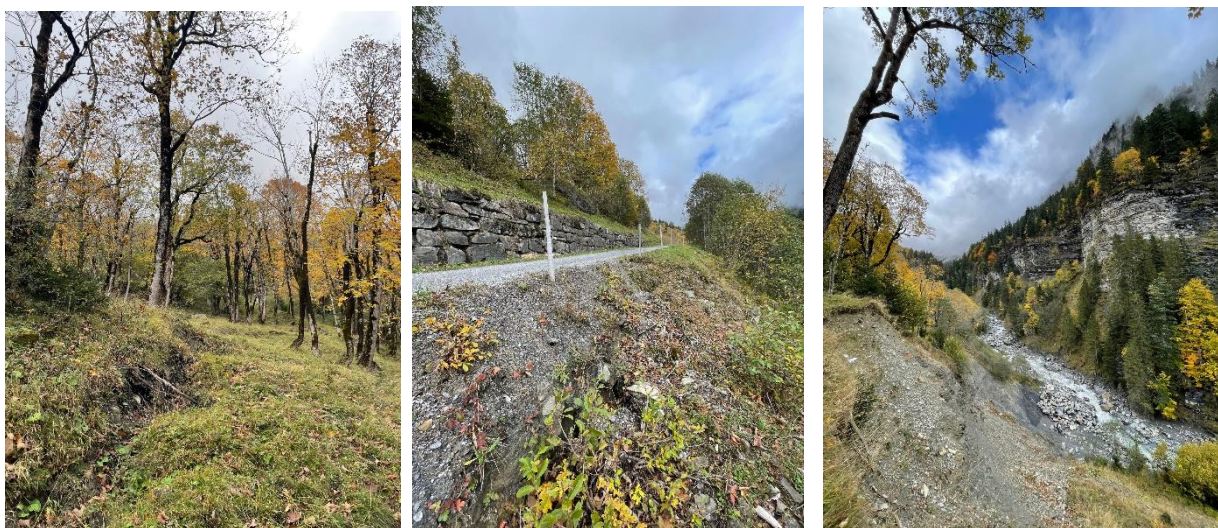
Figure 3: Photographs of visual signs of slope movements: Cracks in the topmost soil layer and tilted trees (left), subsidizing road (middle), and eroded foundation (right).
