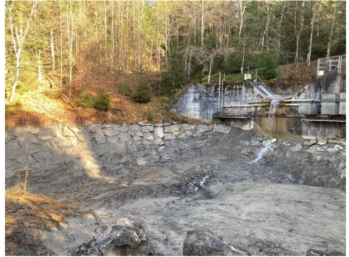
Figure 5. Recently emptied retention basin at the Erlenbach outlet (Source: own photograph, 10.11.25).
