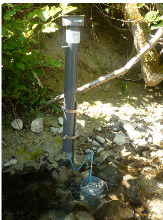
Figure 64 Plug valve of RE WLPWS12 was out of the water after a dry spell of unexpected dimension (Photo: A. Maurer).
