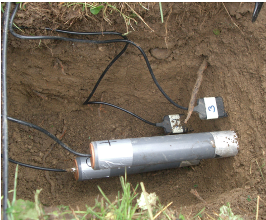
Figure 25: Installation of the water content sensors in the middle hole (10HS on top, TDR on bottom).
