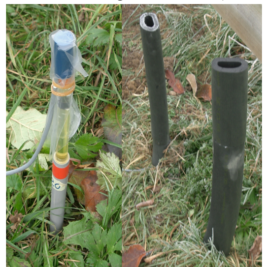
Figure 27: Tensiometer after the installation without (left) and with foam radiation shields (improved version).
