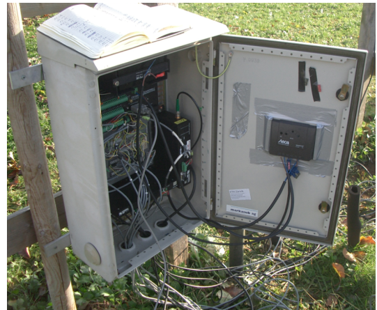
Figure 26: Metal case with data logging system and power supply.
