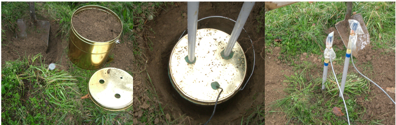
Figure 29: Installation of the lysimeter (from left to right): 1) digging a hole and filling the bucket, 2) insertion of sensors, sealing and placing of bucket in whole, 3) closing hole and complete installation of tensiometers.
