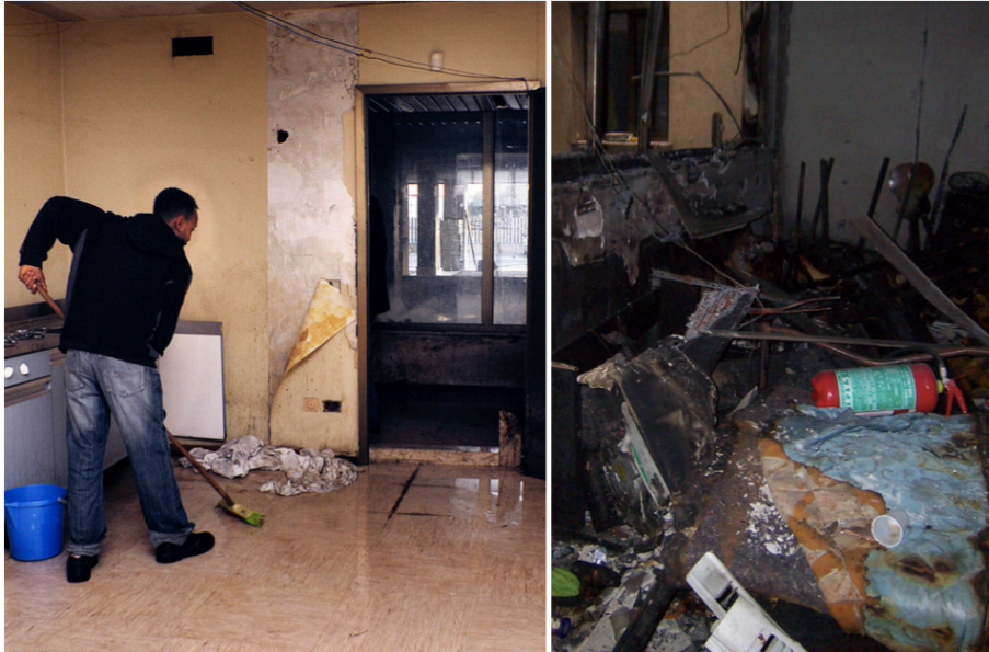
Figure 6: The consequences of the absent maintenance are floods and unfortunately also fire.
