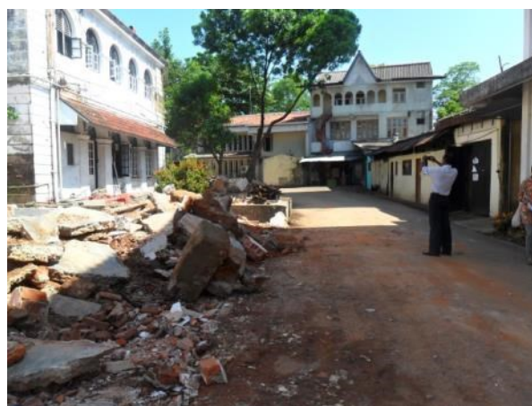
Figure 9: The building complex was dilapidated (Source: UDA, 2014)
