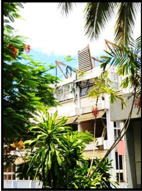
Damage caused by cyclone Pam 2 years on. Port Vila, Vanuatu (Source: self)
