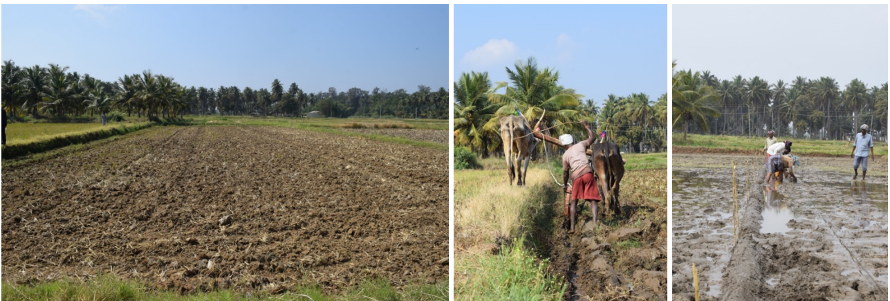
Figure 26: experimental field. Own picture. Figure 27: ploughing. Own picture. Figure 28: wall construction. Own picture.
