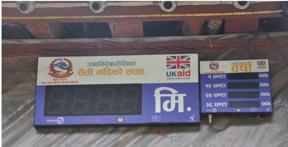
Figure 10: Display and alarm of the EWS in Karuva. (Source: Photo by the author)
