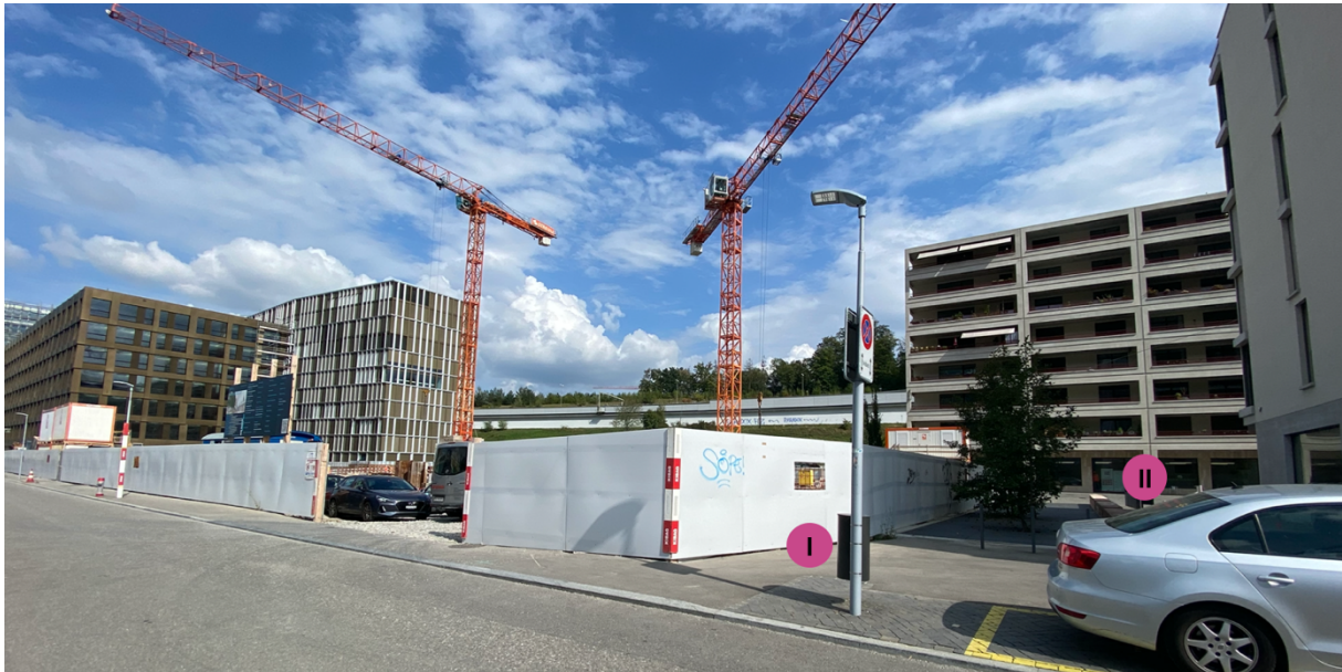
Figure 21: Study locations for estimation tasks (I) and occlusion tasks (II) at construction site of Allmend school building surrounded by white barrier walls.
