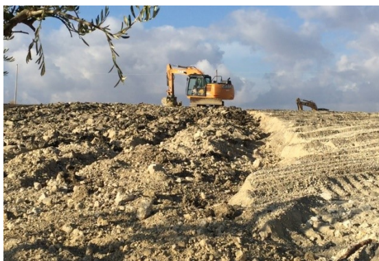
FIGURE 2.1: Soil preparation and rock excavation to produce mineral powder in Sicily (credit: Prof. Dr. Markus Egli).
