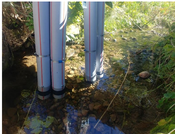
Figure 10: The installation of the stilling tubes in the very calm Rietholzbach.
