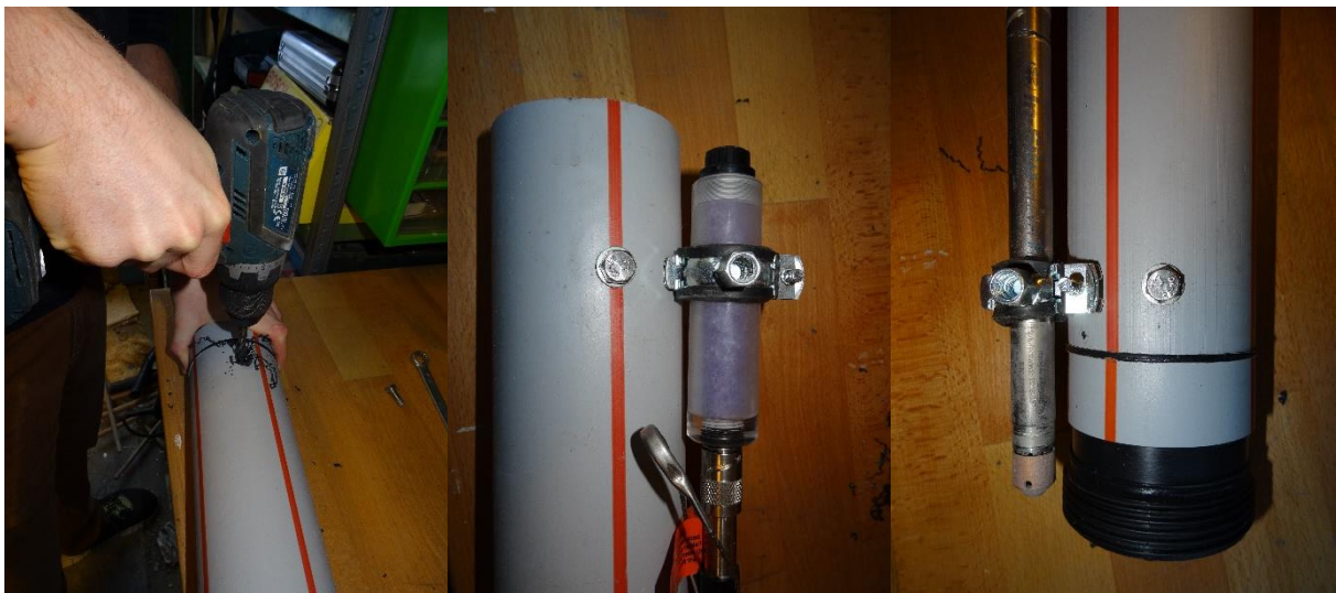
Figure 33: The holes are drilled with a normal drilling machine and an 8 mm drilling bit (left). Afterwards the M8 bolts with a washer fit tightly through the hole (middle and right) and can be connected to the pipe clamps. Also, the pipe clamps can be placed higher or lower on the desiccant and pressure transducer to have an optimal placing of them inside the tube. After the adjustment of the pipe clamps, the desiccant and the sensor are mounted inside the tube.
