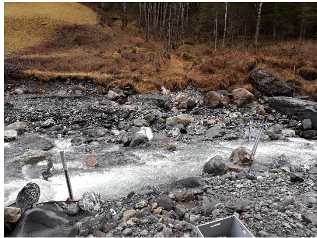
Figure 17: The installation of the stilling tubes in the Untertalbach. The reference tube and the tube filtered with the G1/4" thread and O-ring filter are mounted to the stake in the front right, the tube with the G1/2" thread and O-ring filter in the front left and the tube with the G1/8" thread and O-ring filter on the other shore in the back.
