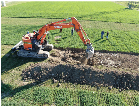
(A) Mechanical loosening of the soil with a digger (Photo: Alice Johannes).
