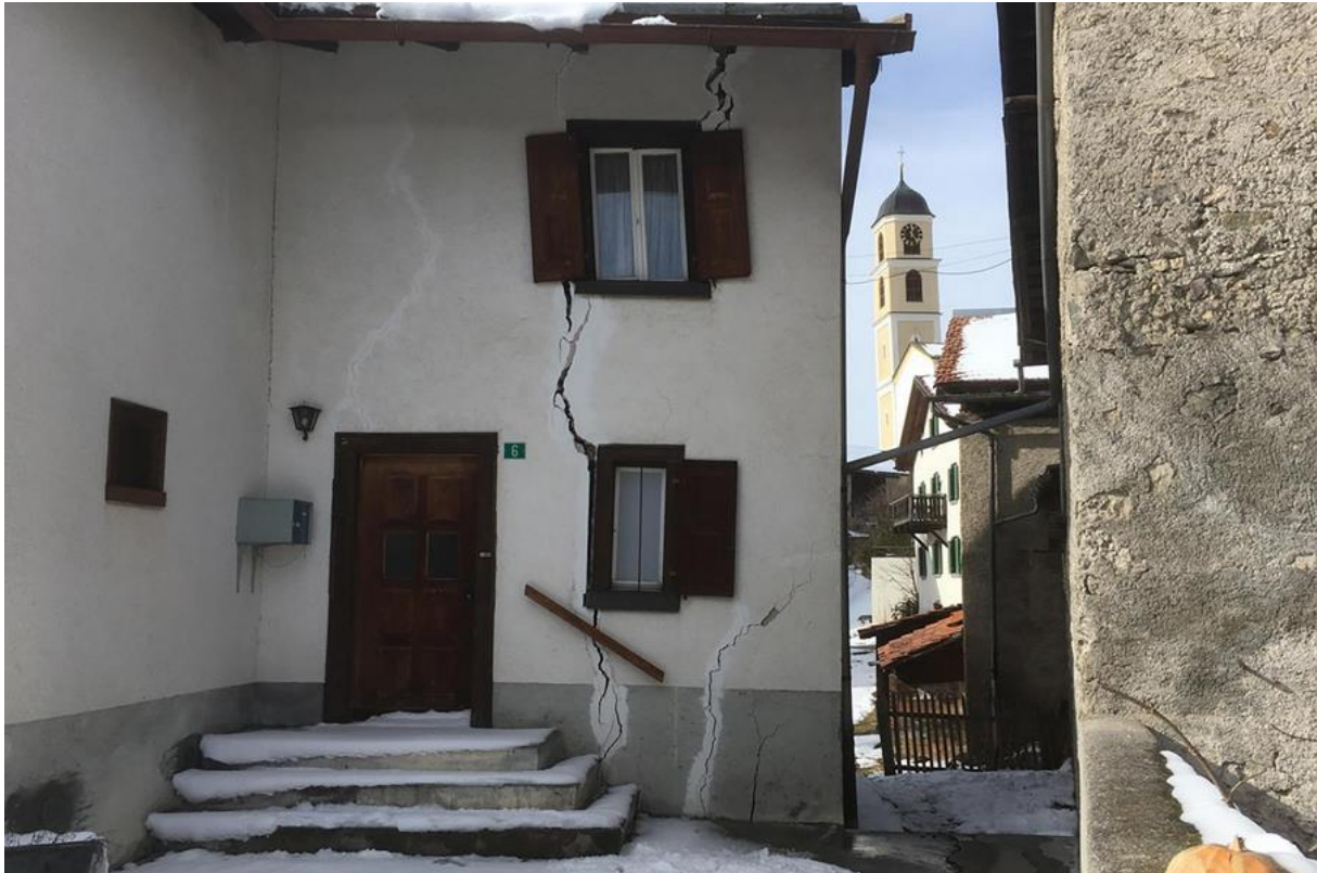
Fig. 21: The houses in Brienz/Brinzauls GR are damaged by the slide and the church tower stands lopsided. Source: Lukas Denzler.
