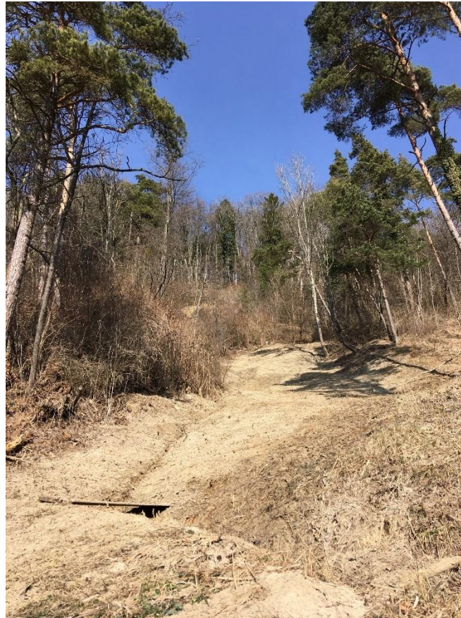
Figure 3: Westernmost reach of the Diebisbach, Switzerland, under construction (photo by M. Steinmann, 2018)
