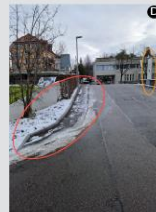
Figure D: Pavement non compliant, too narrow and no low curb (ellipse red) and no complete information board (ellipse orange)
