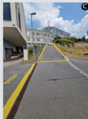
Figure C: Standard compliant gradient (yellow trapezoid), but challenging for wheelchair users and no safety railing (ellipse orange) to the meadow
